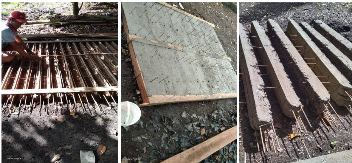
Fig.32. Framing and production of concrete post for fencing in DA-Aroman, North Cotabato and JRMSUTampilisan Campus.
